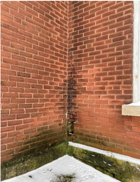
Plate 31: Location of former downspout on east elevation
