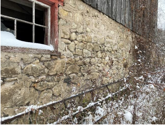
Plate 41: Barn fieldstone foundation
