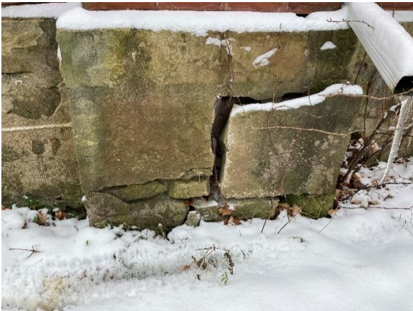
Plate 27: Deterioration in the foundation of the west chimney on the west elevation
