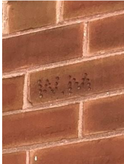
Plate 32: Detail showing W.M. graffiti on east elevation
