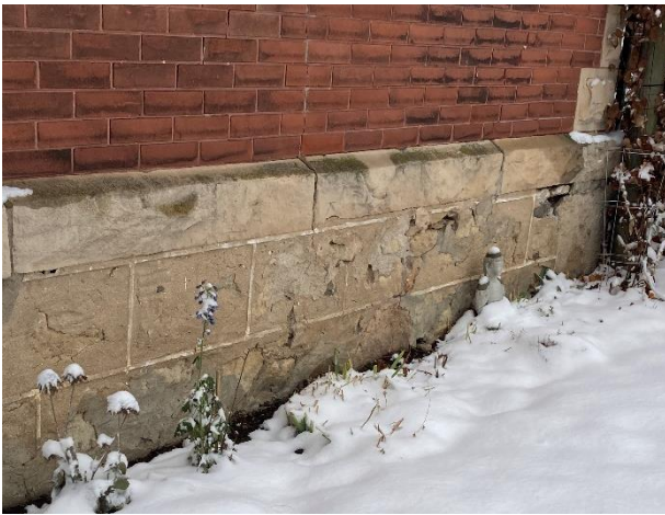
Plate 19: Parged stone foundation
